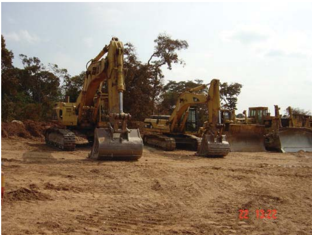
PHOTO 2. KAMAKANGA MINING PLANT, PART OF THE ASSETS ACQUIRED BY GEMFIELDS
